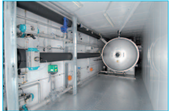
Ozone generator and pipework installed in container
