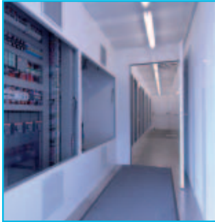
The inside of the container showing the electrical power supply and control equipment
